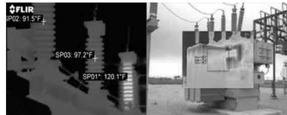
Fig. 4: Thermal View of Internal Inspection of Substation equipments
